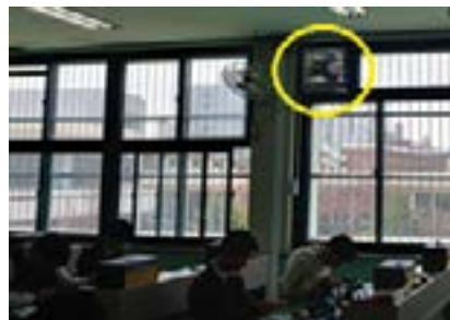
Insufficient ventilation system in a soldering lab
